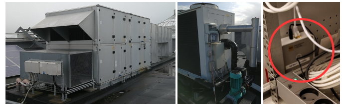
Fig. 1. From left; AHU, chiller unit and Building Management System (BMS) gateway for remote data acquisition and control, situated at Kolding Storcenter, a Danish shopping center.
