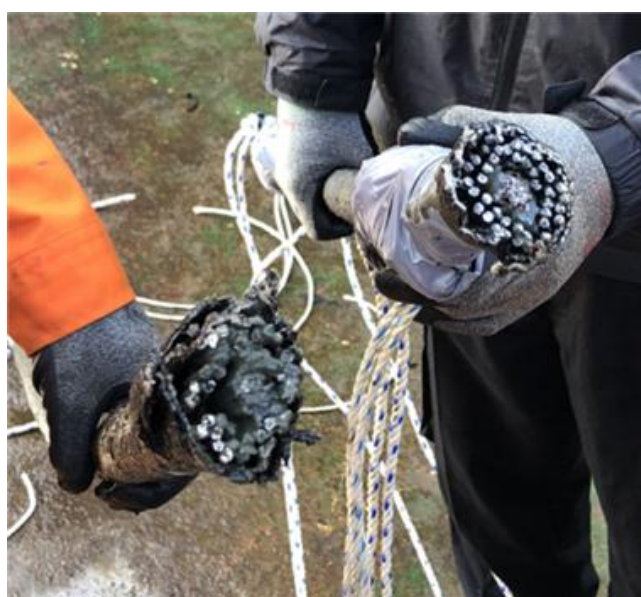
Fig. 15. Cable cut by cutting tool
