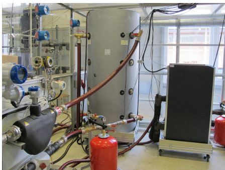
Fig. 1. Testbed with heat pump (right), storage tank, circulation pump (middle) and heat meter (left)
