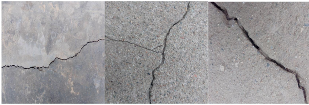
Fig. 9. Partial sample image of bridge crack data set
